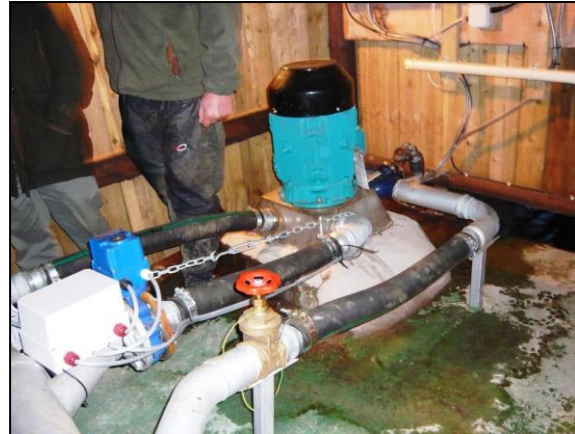
Inside the pump house at Auchencheyne.
