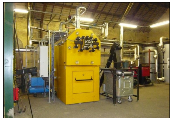
Woodchip boiler at Floors Castle. Hot water accumulator tanks far right. Silver wheeled skip for ash removal.
